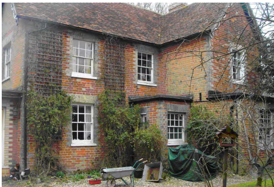
Picture 1.14 Trevor House Windows and other selected architectural detailing which may be protected by an Article 4 Direction subject to further consideration and notification
