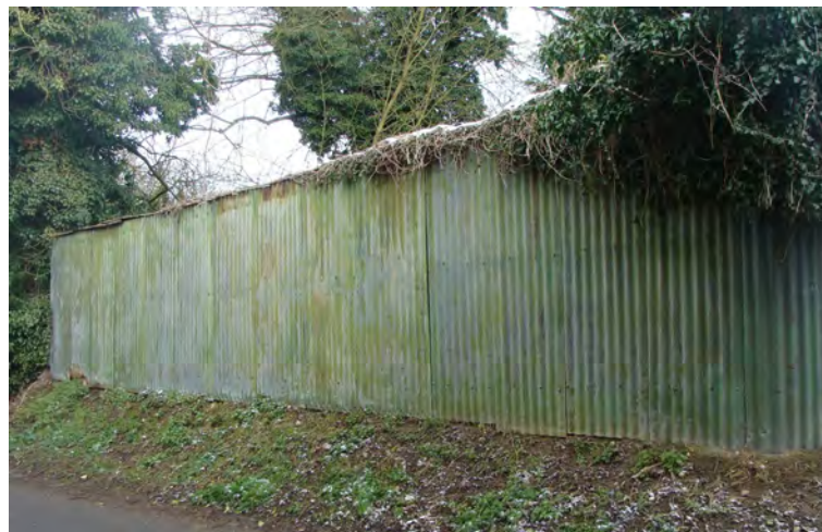
Picture 1.23 Corrugated structure adjacent to Church Hill, north side. Ideally needs replacing but if remaining there is potential to explore planting of native hedge species to front
